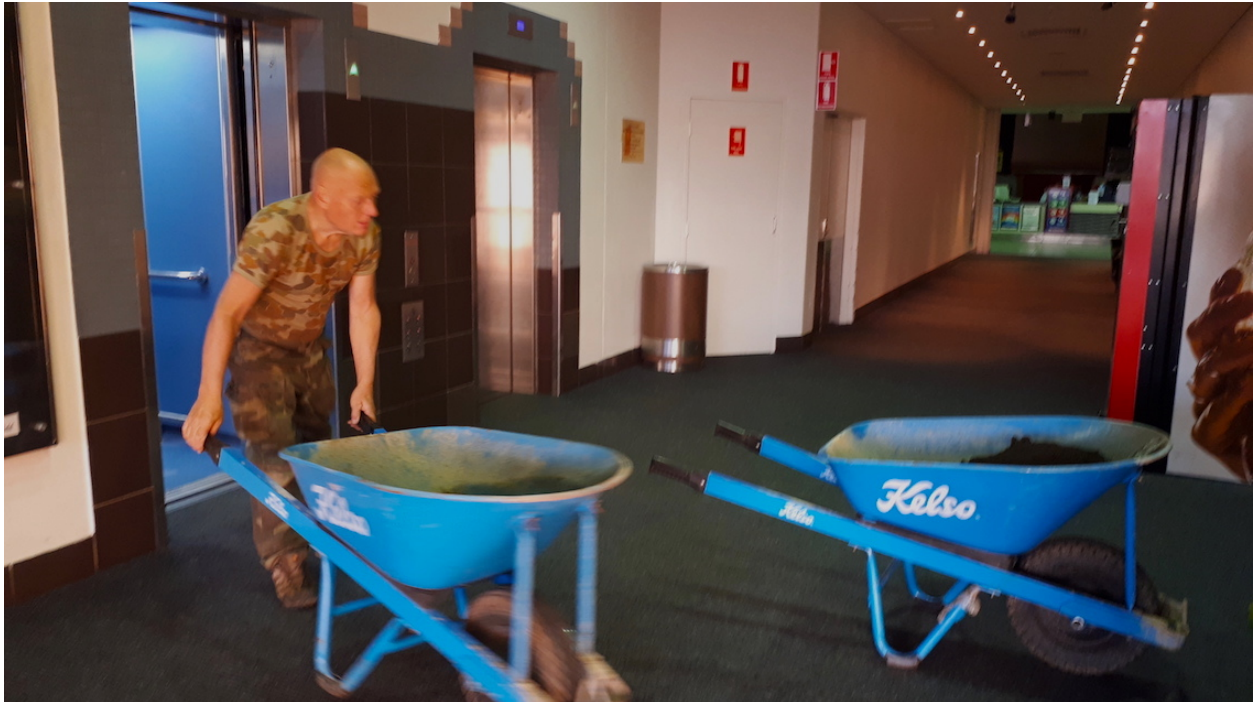
Swapping an empty wheelbarrow for a full one. Precision timing with the lift doors.
